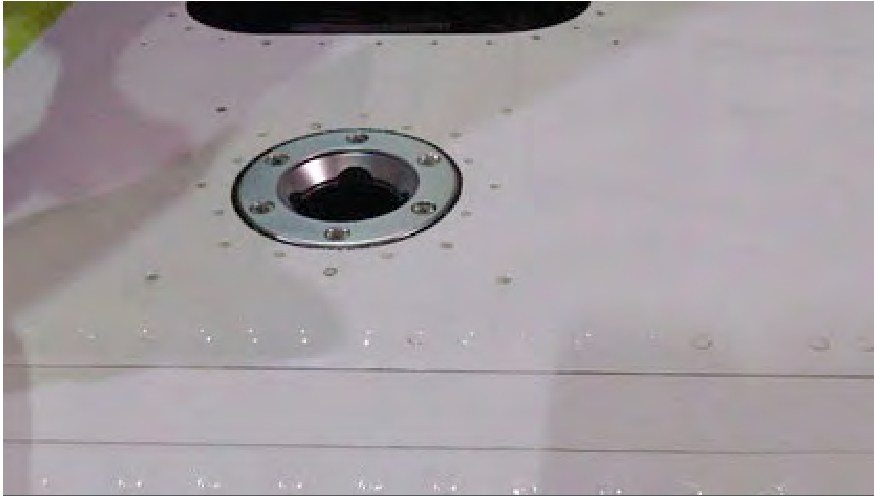
The bladder is inserted into the wing and the filler neck is installed.
