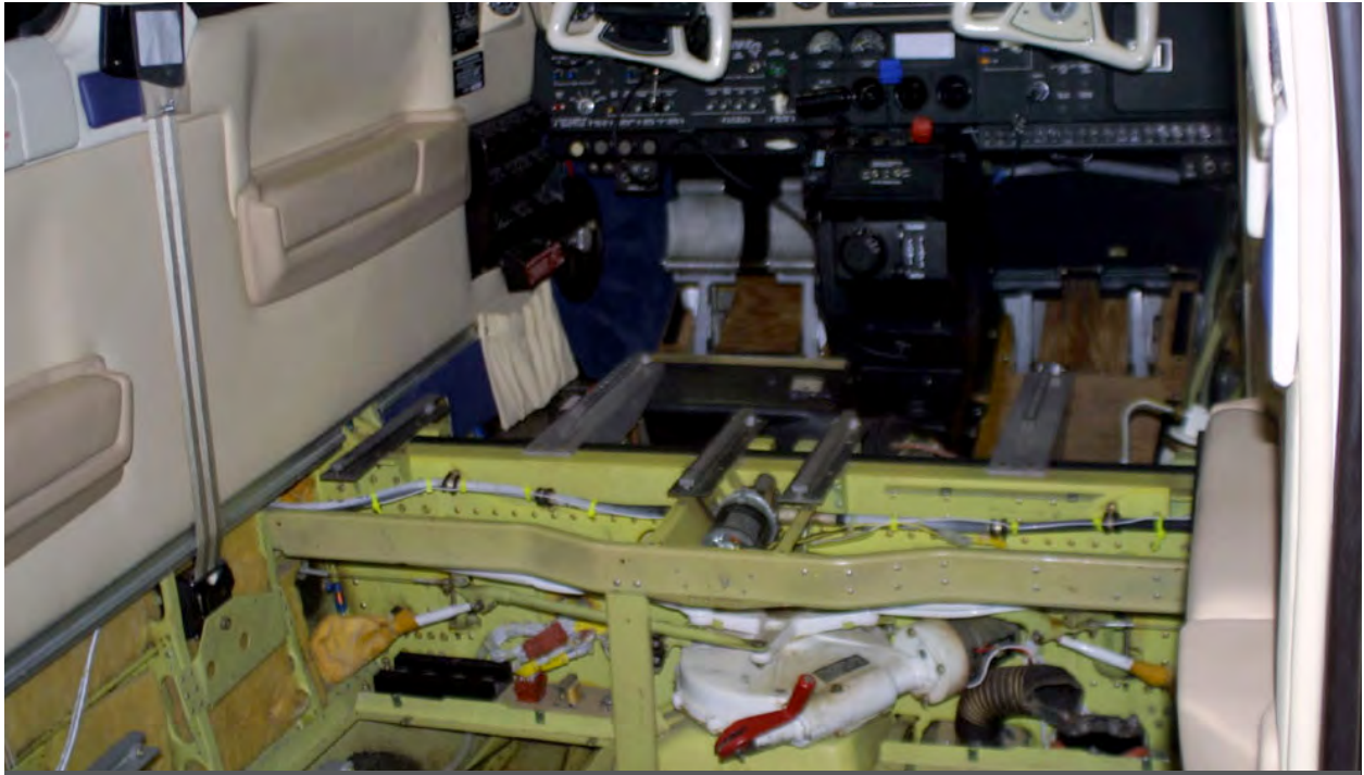
The interior is stripped to give the installer access. Plumbing will be routed throughout.
