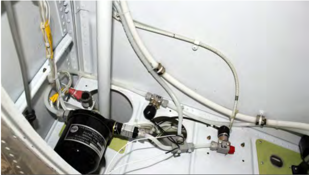
The TKS filter, low pressure switch, high pressure switch and main pumps are located in the wheel well looking outboard.
