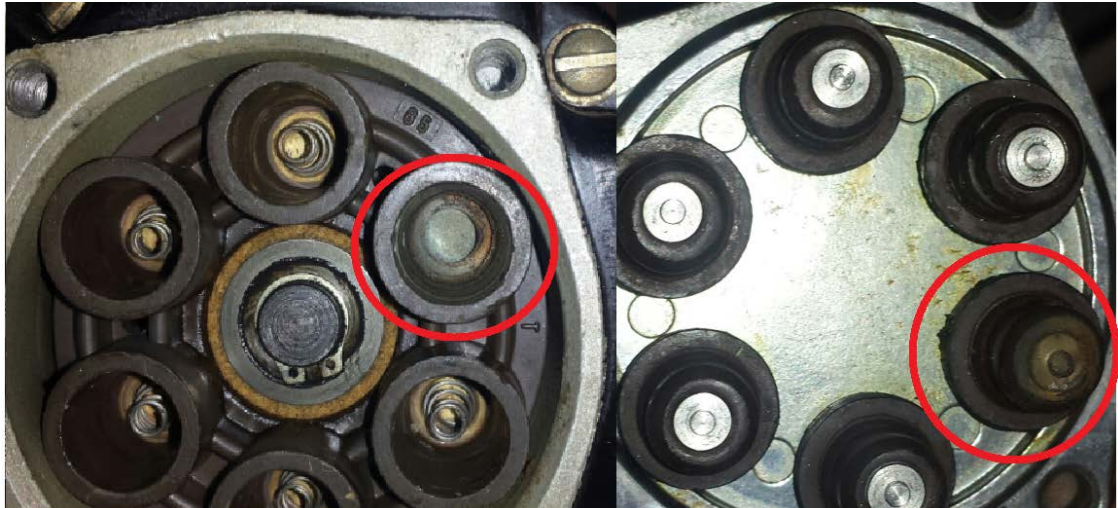
Figure 12 - Missing block spring
